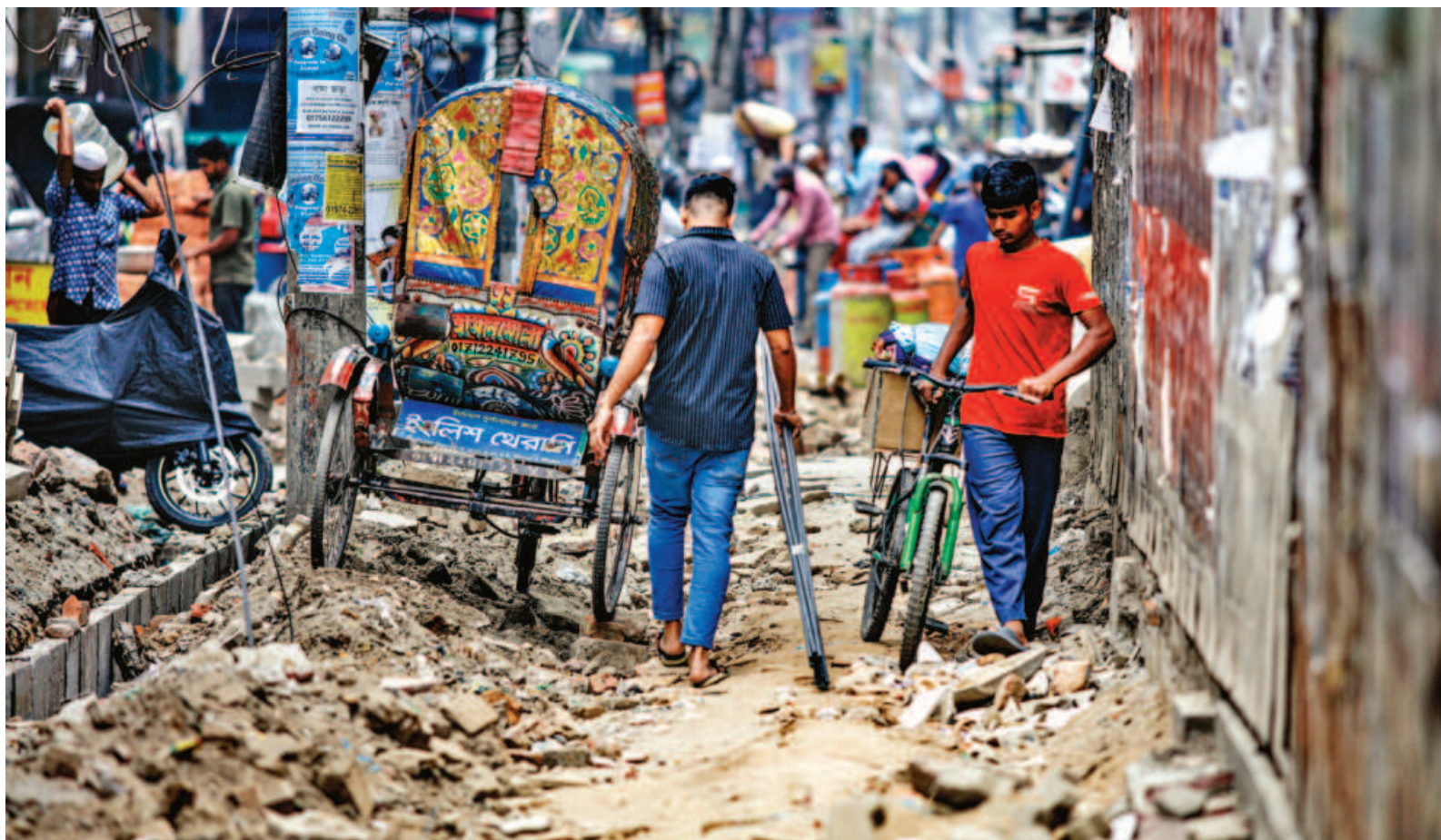
Ongoing pavement renovation by Dhaka South City Corporation under the Moghbazar flyover has put pedestrians in trouble. They have been struggling to walk as rickshaws frequently park on the pavement, while cyclists often use it to bypass traffic. The pavement has been in this state for 10 days. This photo was taken yesterday.
