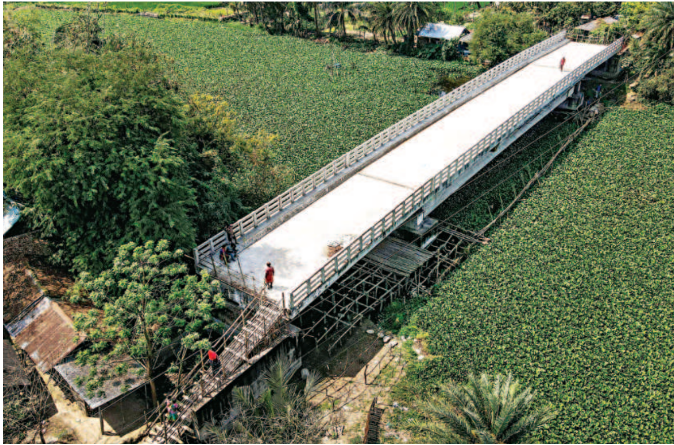
Construction of the bridge in Badurgacha area of Dumuria, Khulna, was completed eight years ago. But the only way to access the bridge is the rickety staircase made of bamboo and wood as the authorities could not build roads because they had not acquired land on either side of the structure.
