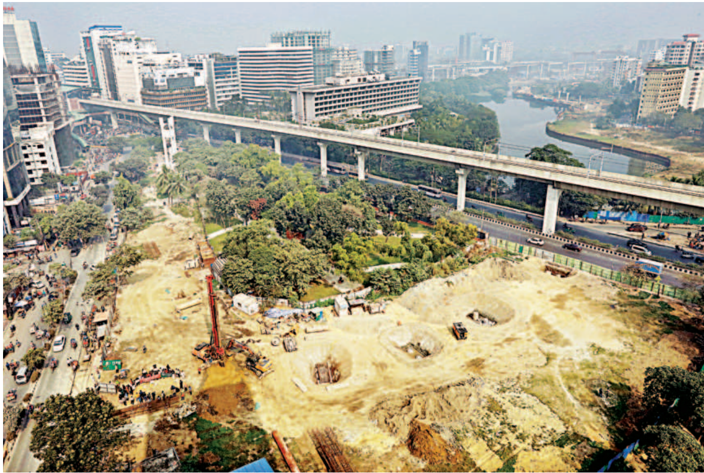
Construction work is going on at the Panthakunja Park near Sonargaon intersection in the capital. Bangladesh Gacch Rakkha Andolon demonstrated at the park yesterday demanding cessation of the construction work for an elevated expressway ramp that they said would destroy park. PHOTO: AMRAN HOSSAIN
