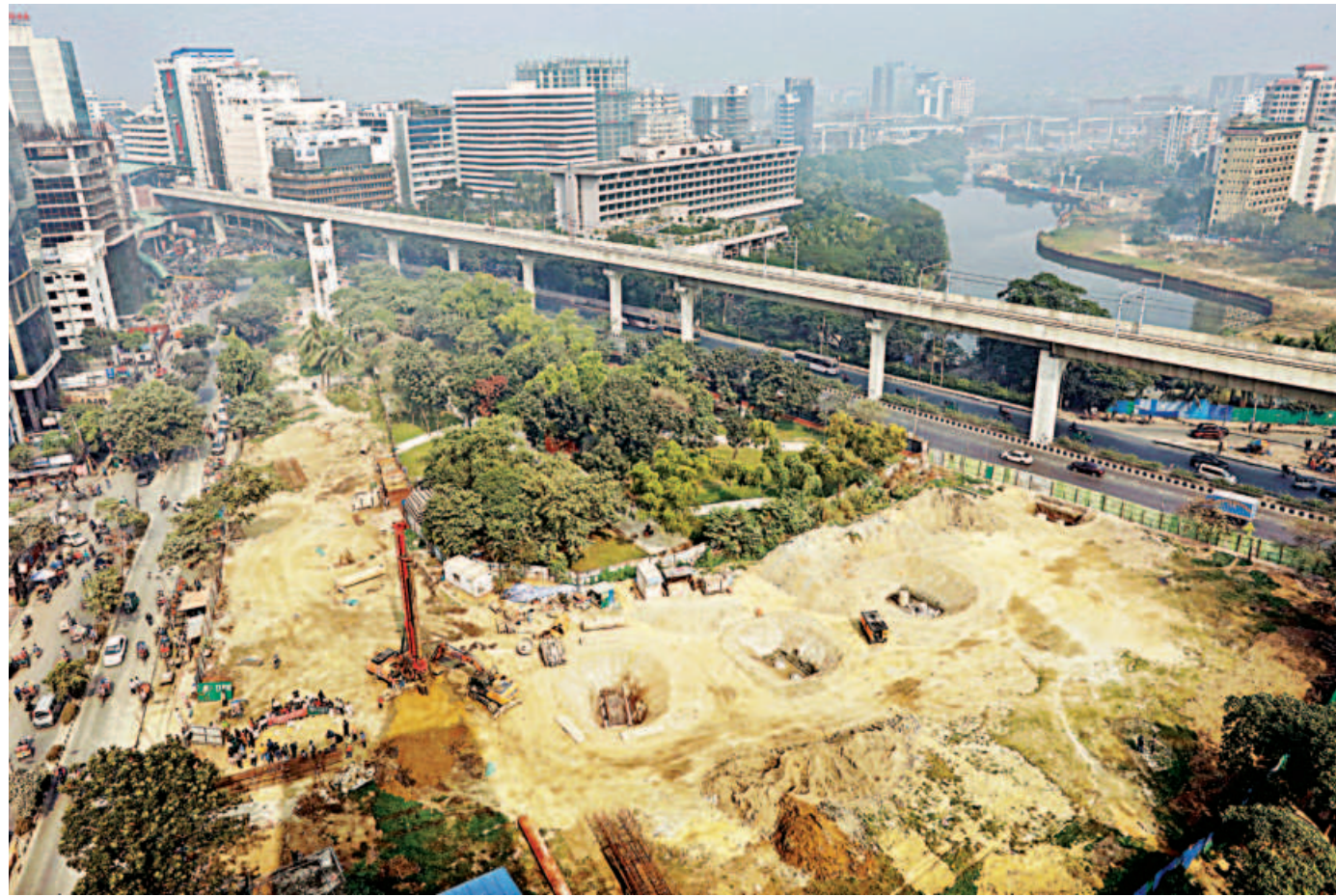
Construction work is going on at the Panthakunja Park near Sonargaon intersection in the capital. Bangladesh Gacch Rakkha Andolon demonstrated at the park yesterday demanding cessation of the construction work for an elevated expressway ramp that they said would destroy park.
