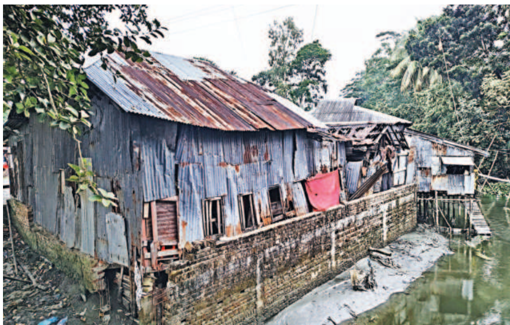
Basugi canal has been reduced to a narrow ditch filled with dark, polluted water and almost no flow due to the accumulation of solid waste and encroachment.
