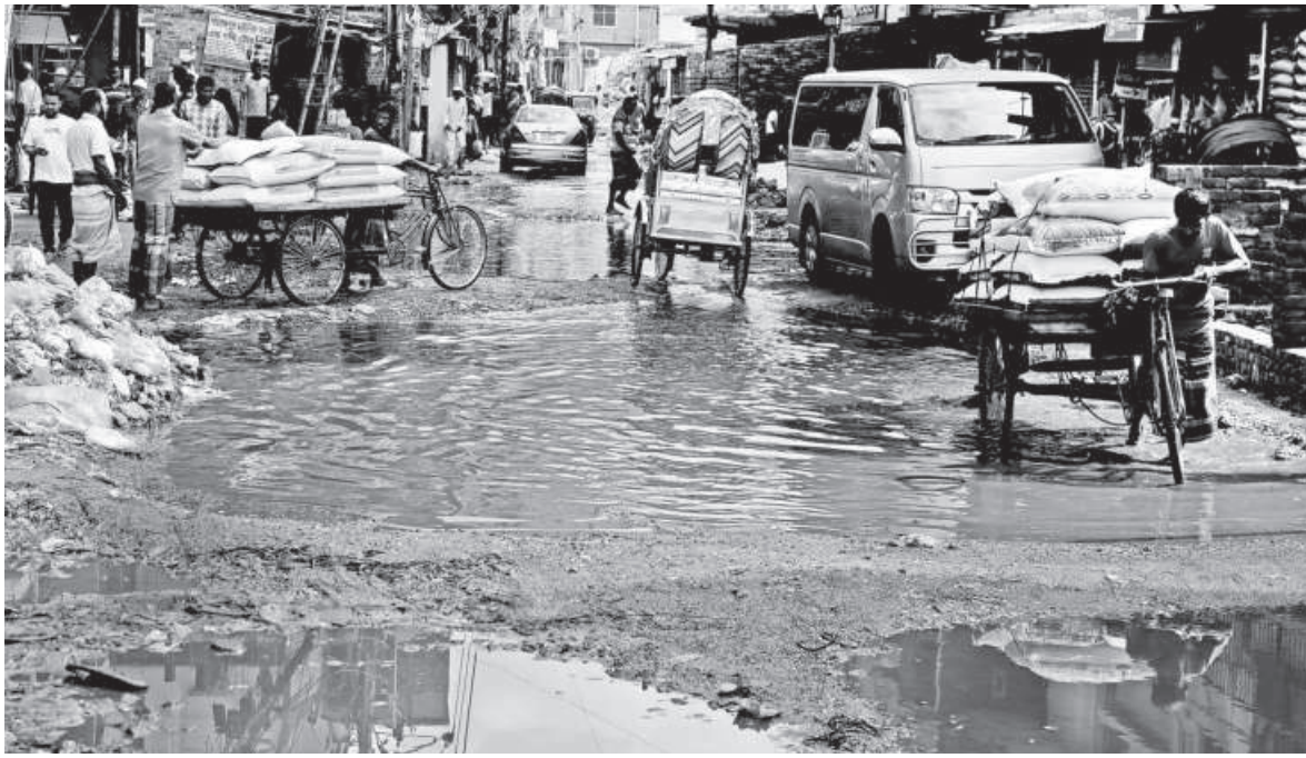
Water accumulates in these potholes whenever it rains or if the drain overflows. Following heavy rains earlier, these potholes were formed and are yet to be fixed. In the meanwhile, they continue to be a nuisance for pedestrians and vehicles. The photo was taken in the Manda area recently.
