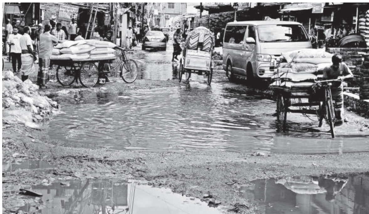
Water accumulates in these potholes whenever it rains or if the drain overflows. Following heavy rains earlier, these potholes were formed and are yet to be fixed. In the meanwhile, they continue to be a nuisance for pedestrians and vehicles. The photo was taken in the Manda area recently.
