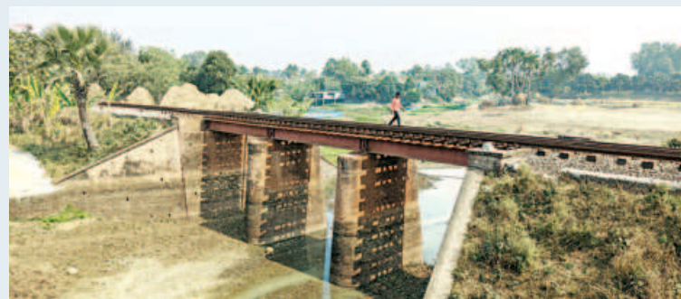
Present photo of Sahagola Bridge in Atrai upazila, Naogaon. Part of the bridge was demolished during an operation on Sept 6, 1971. An incoming Pakistani train was derailed, and over 100 enemy soldiers were killed in a subsequent gunfight.
