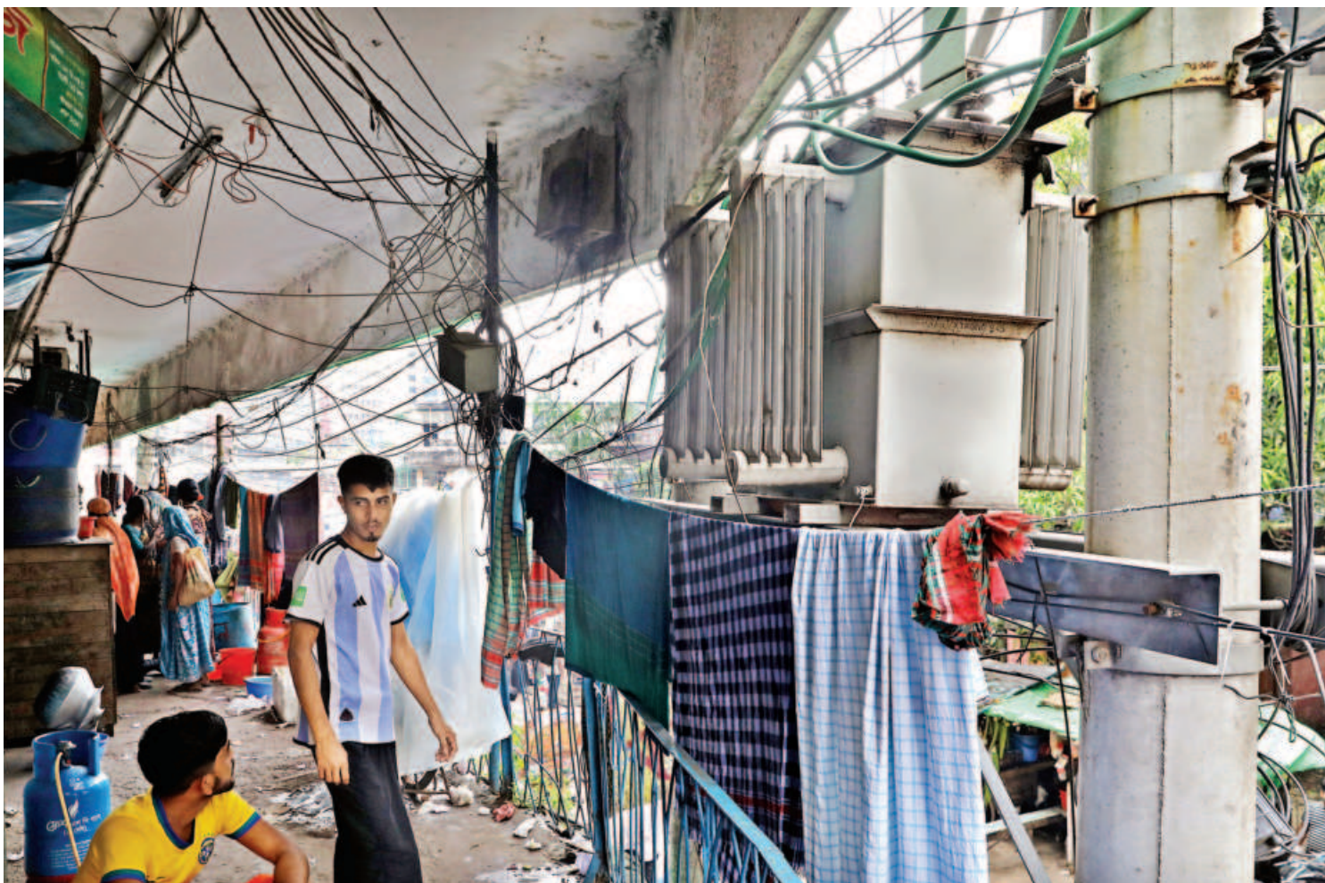
People hang wet clothes right next to this electric transformer for drying. This puts people who use this path at risk of electrocution. The photo was taken in the Kawran Bazar Municipality Market recently.
