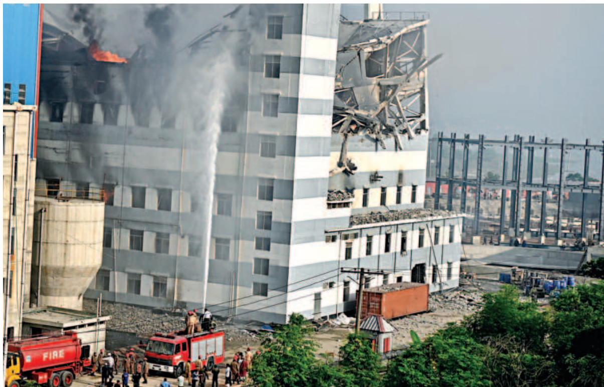
Firefighters tackle a blaze at a tissue factory owned by Meghna Group in Jhauchar area of Narayanganj's Sonargaon upazila yesterday. Fire service officials said the building tilted and two floors collapsed due to intense heat.
