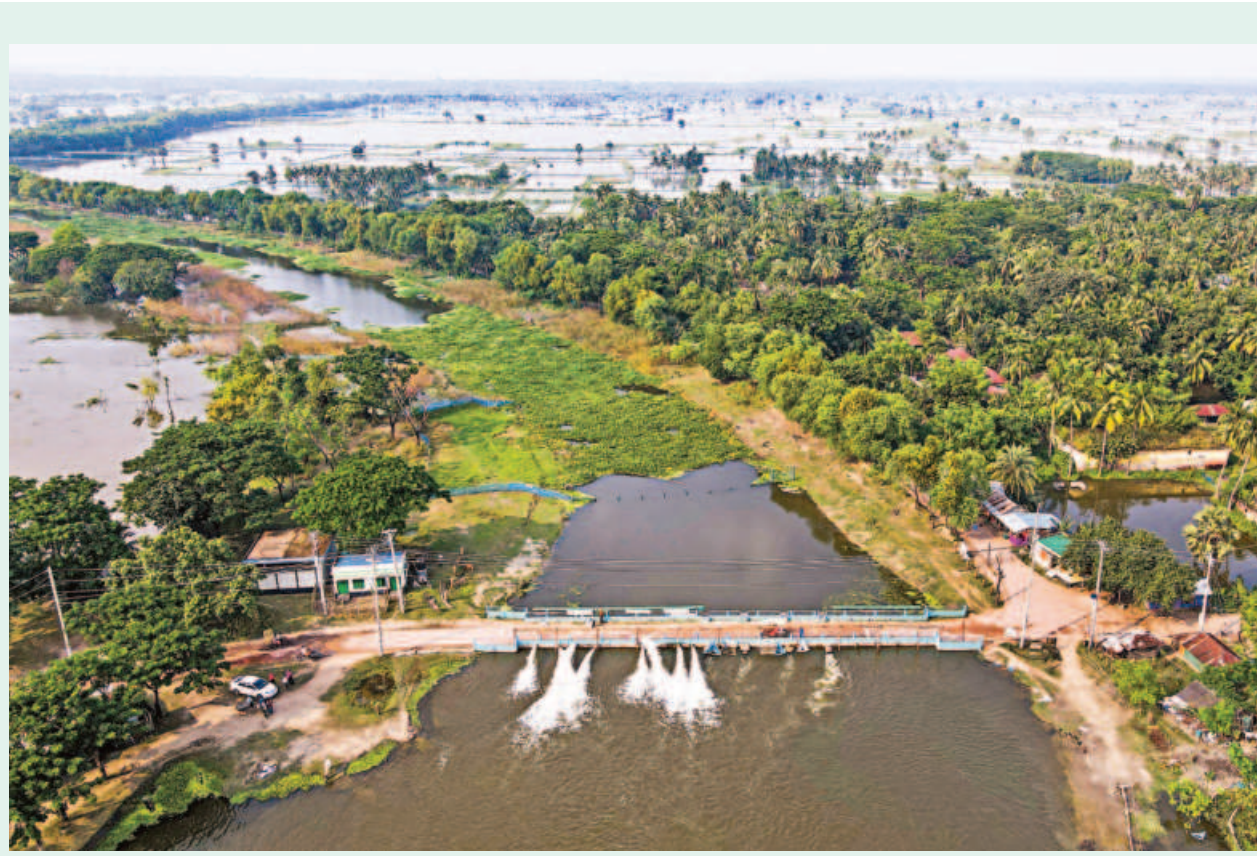
As the Bhabadah 21-vent sluice gate remains non-functional, the pumps installed nearby have to drain out the water from several hundred villages of Jashore and Khulna, which have been suffering from waterlogging for the past two months. However, the pumps are proving to be less effective due to the huge amount of water to pump out. PHOTO: HABIBUR RAHMAN
