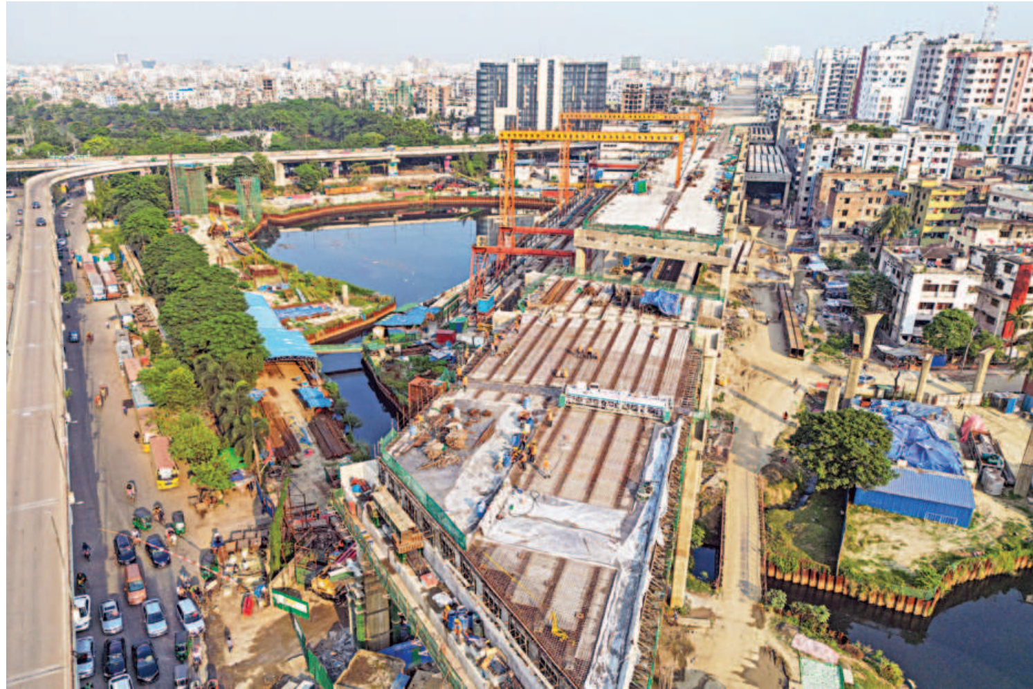
Work on the Dhaka Elevated Expressway resumes near FDC in the capital after a dispute over shares between the private partners of the public-private project halted work for over nine months. The photo was taken yesterday.
