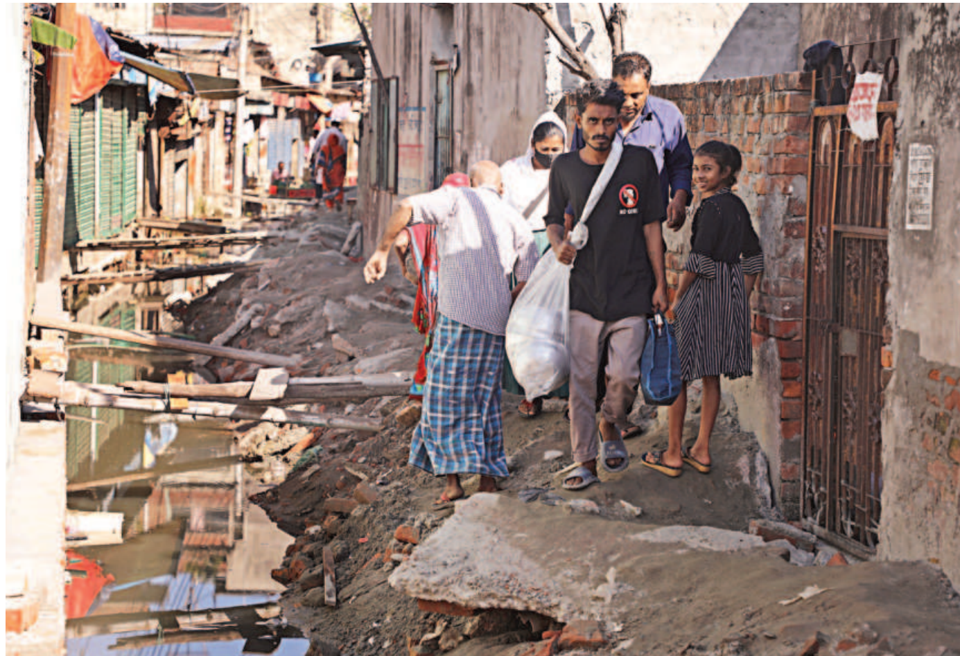
A trench has been dug into Jurain Medical Road in the capital for a sewer line, leaving little room for pedestrians to walk. The road has been left in such a state for about a month. The photo was taken yesterday.
