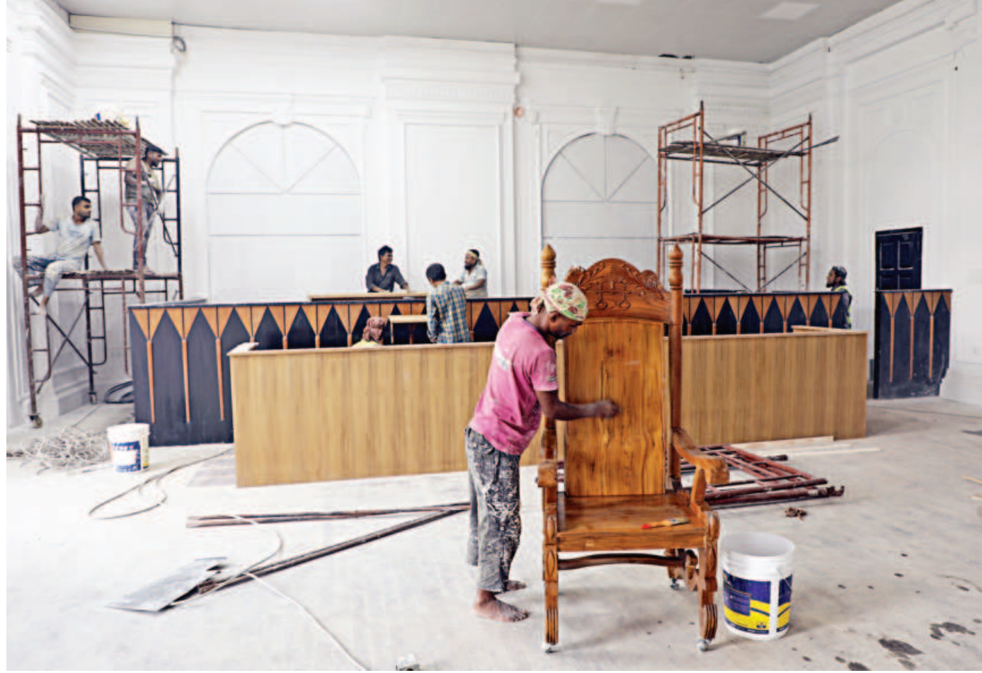
Workers renovating a courtroom for the International Crimes Tribunal where proceedings would begin from November 3 of cases filed over crimes against humanity and genocide during the mass uprising.
