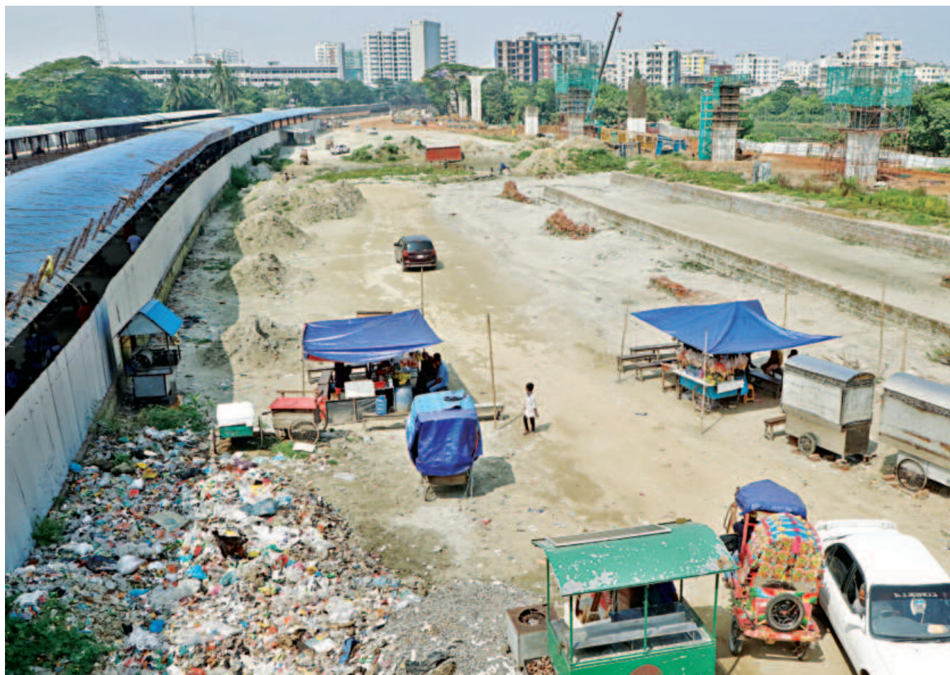
The waterbody adjacent to the Airport Railway Station was filled up six months ago as part of the Dhaka-Tongi-Joydebpur railway expansion project by the Bangladesh Railway. The photo was taken yesterday.
