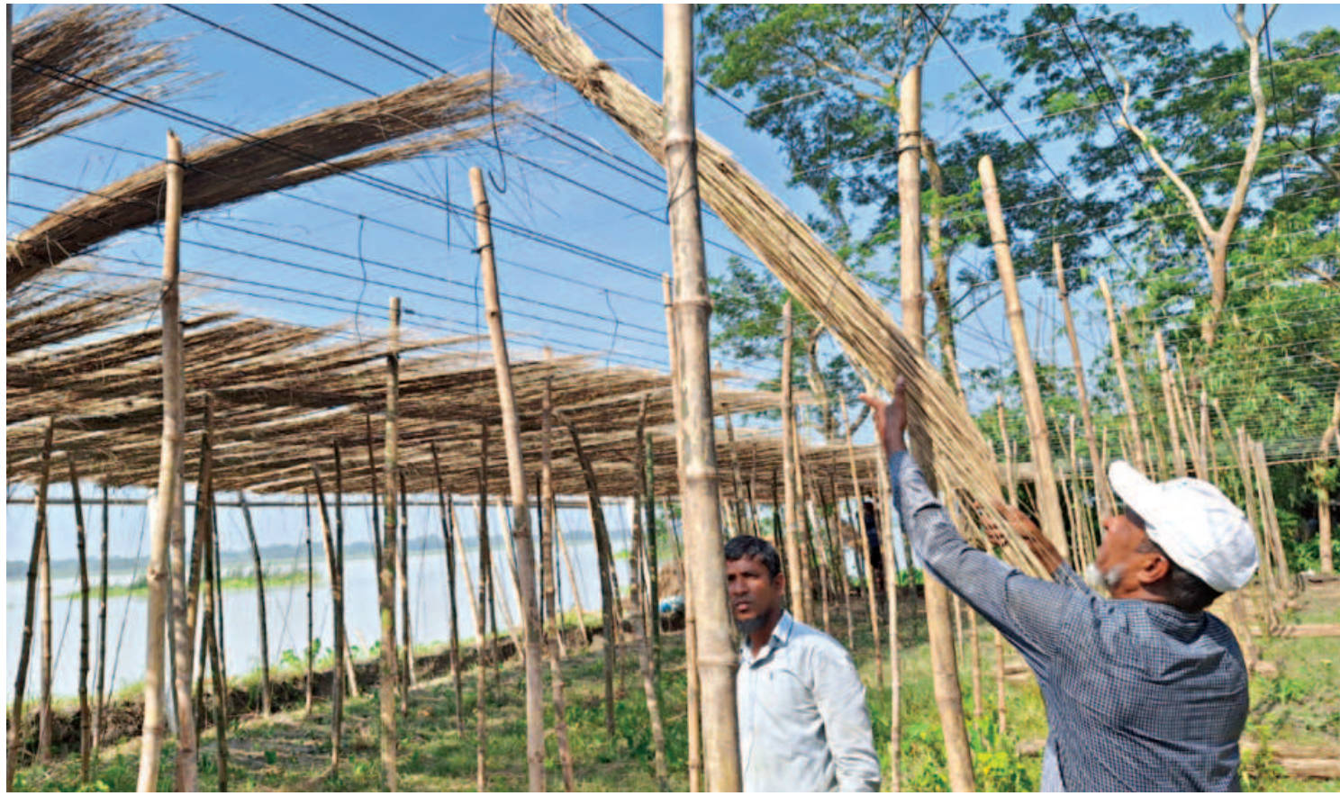
Farmhands are seen laying thatch on a trellis to create shade for the cultivation of betel leaf plants underneath. Each farmhand can earn up to Tk 600 a day working from 8:00am to 3:00pm. The picture was taken at a farm in Wazirpur upazila of Barishal district recently.
