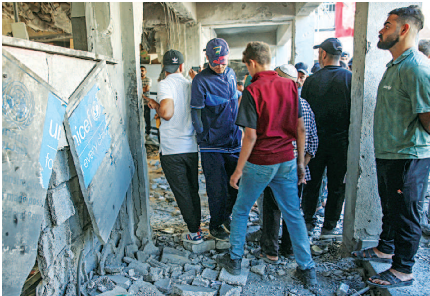
Displaced Palestinians check the damage inside a UN school-turned-refugee in the Al-Shati refugee camp near Gaza City in the northern Gaza Strip, following an Israeli strike yesterday.
