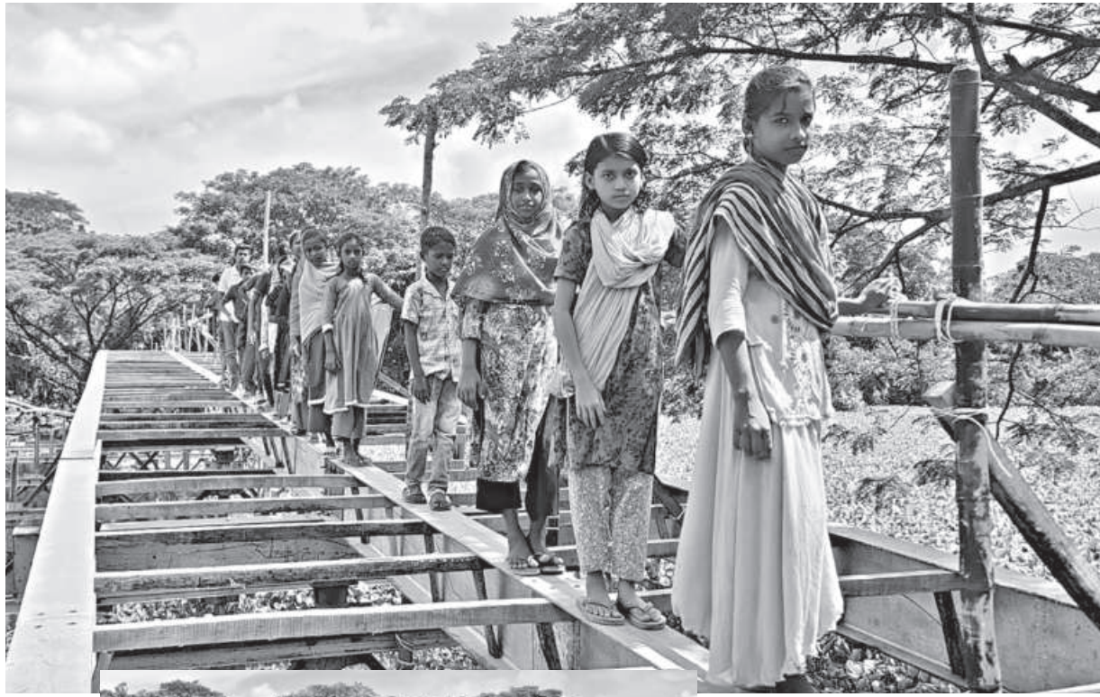
Risking lives, children cross an incomplete bridge over Madarbunia Canal in Patuakhali's Rangabali upazila. Even though more than a year has passed since stipulated deadline of the construction work, the bridge lies unfinished. The photo was taken recently.
