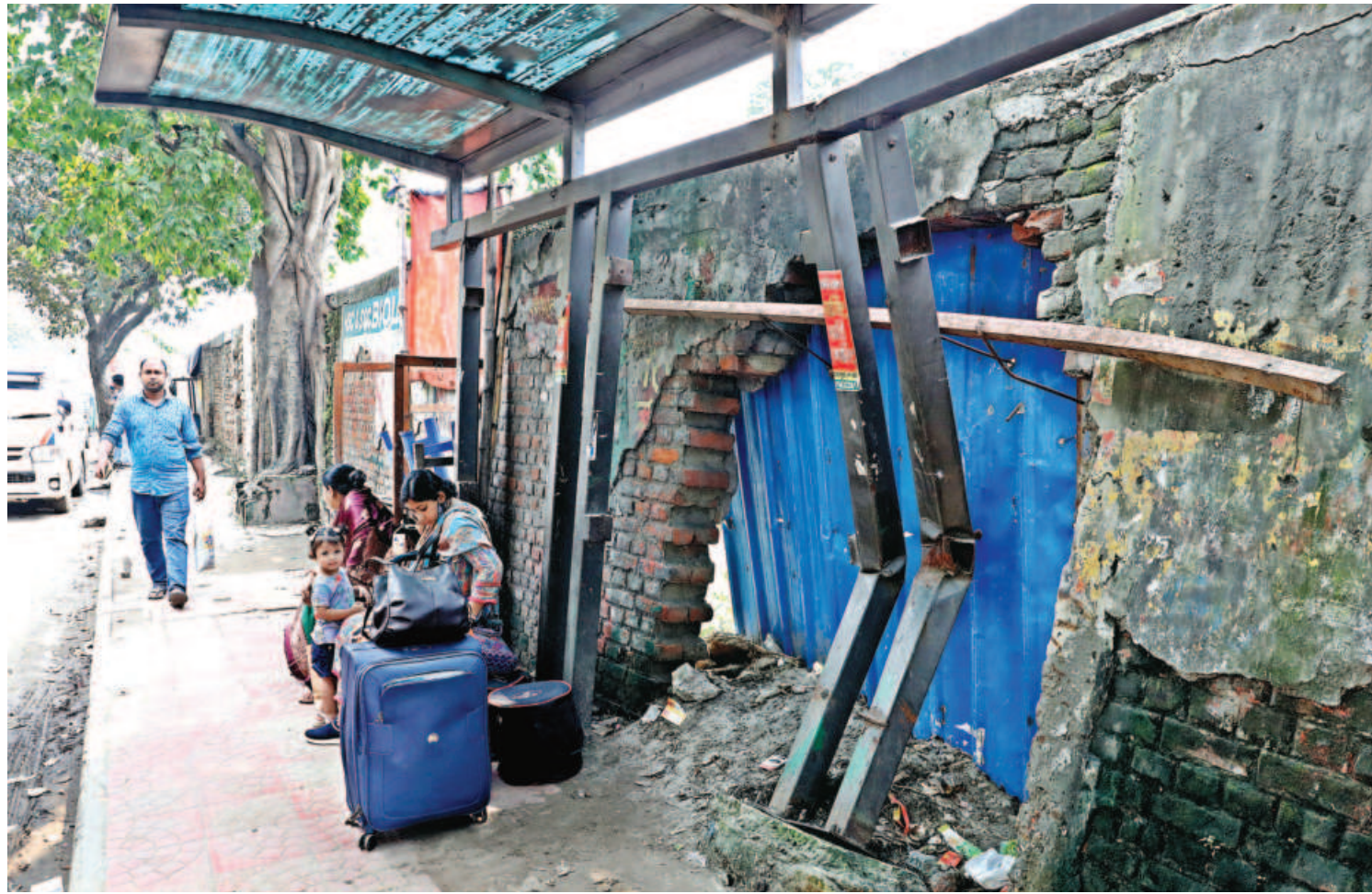
A group of people waiting under a crumbling passenger shade in the Basabo area of Dhaka yesterday. The rusted beams and partially collapsed wall, barely held together, pose a serious risk of collapse. With cracks and exposed metal, the structure is a potential hazard for those waiting underneath, raising concerns that an accident could occur at any moment if repairs are not made promptly. PHOTO: ANISUR RAHMAN
