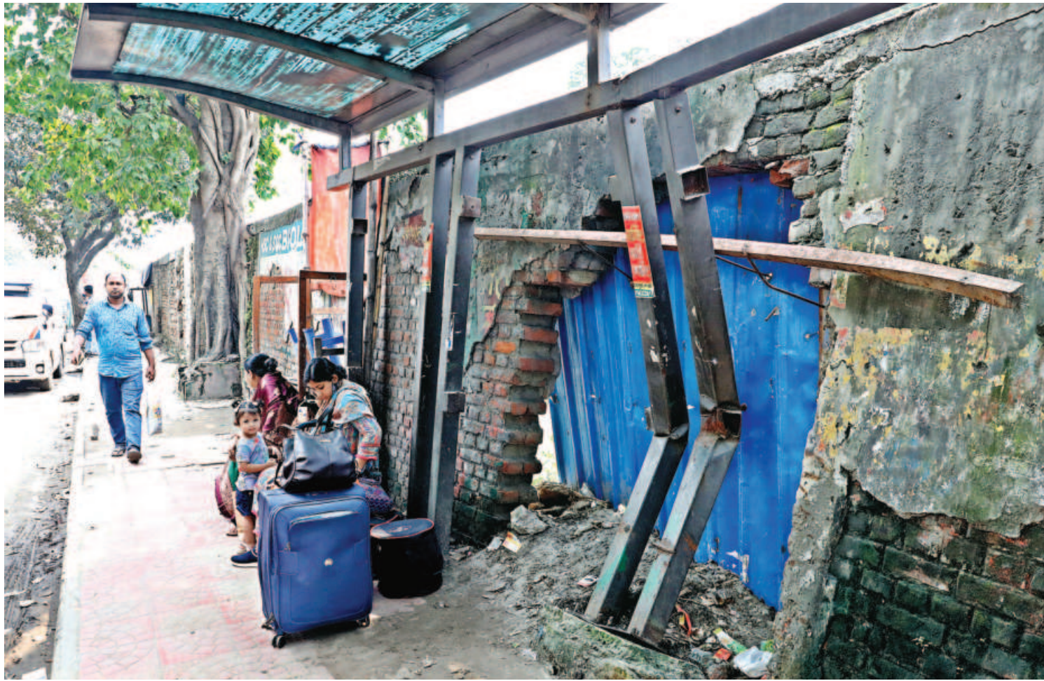
A group of people waiting under a crumbling passenger shade in the Basabo area of Dhaka yesterday. The rusted beams and partially collapsed wall, barely held together, pose a serious risk of collapse. With cracks and exposed metal, the structure is a potential hazard for those waiting underneath, raising concerns that an accident could occur at any moment if repairs are not made promptly. PHOTO: ANISUR RAHMAN
