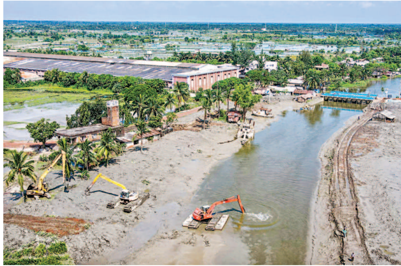
Silt accumulated near the Sholmari river sluice gate being removed by excavators. The river acts as the only means of water drainage for hundreds of villages in Khulna's Dumuria upazila. With so much silt near the gate, the villages have been facing intense waterlogging since the beginning of the monsoon. The photo was taken recently.
