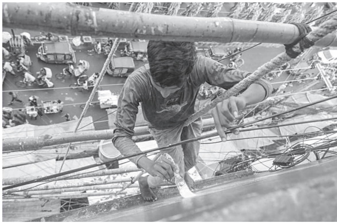
With no safety gear on, a construction worker paints a high-rise building in New Market area of Chattogram city yesterday. While deaths and injuries of such workers are common occurrences in the city and elsewhere, no substantial measures are visible in ensuring their occupational safety.
