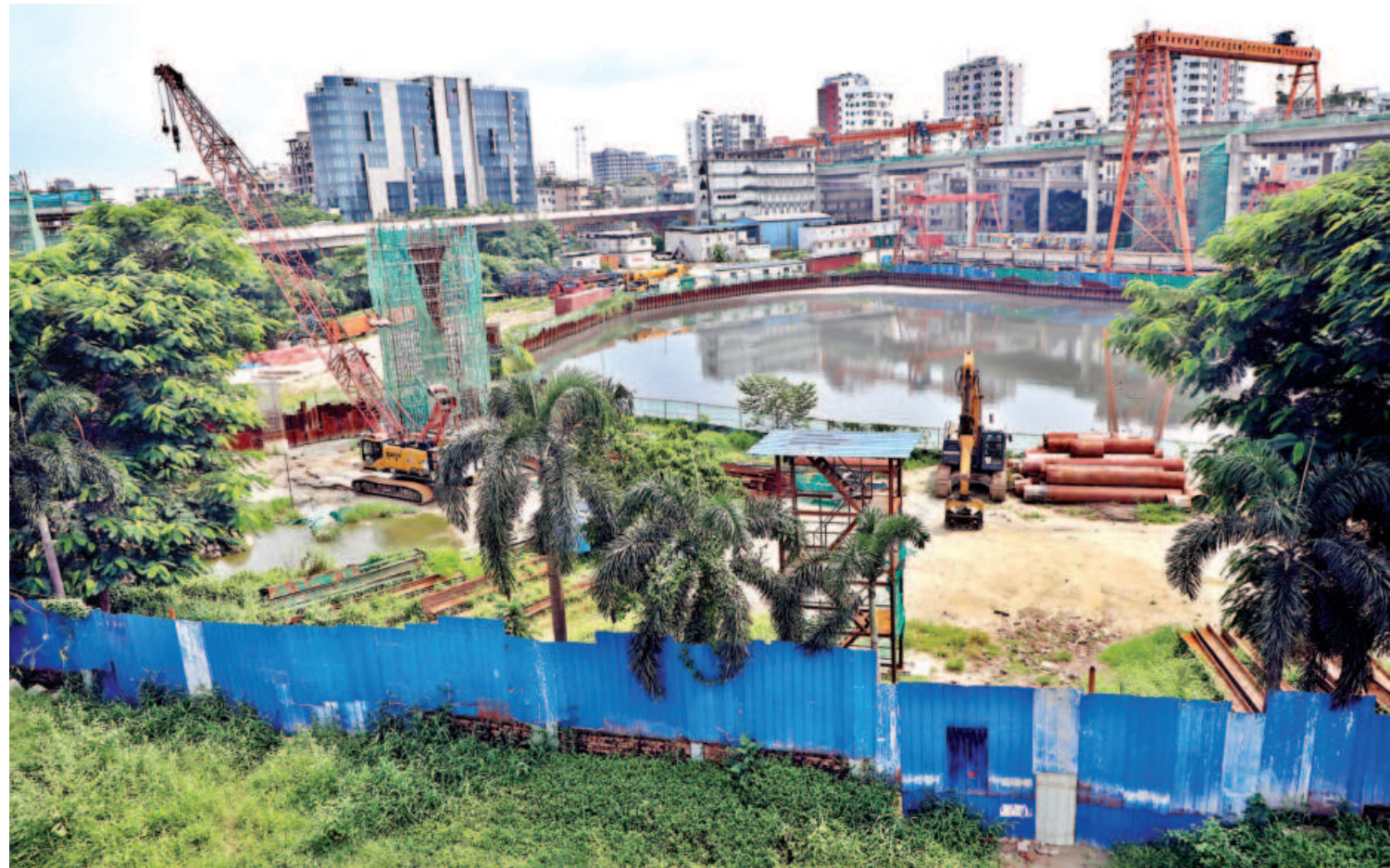
Large pillars and scaffolding rise from what was once a part of Hatirjheel. Over 10 acres of the waterbody has been filled with sand as part of the Dhaka Elevated Expressway. Cranes, excavators, and now temporary offices occupy the site. The place has been cordoned off with barricades. Authorities claim the filling was necessary to construct 41 pillars for the expressway, but environmentalists warn this could exacerbate the city's waterlogging woes. The photos were taken yesterday.
