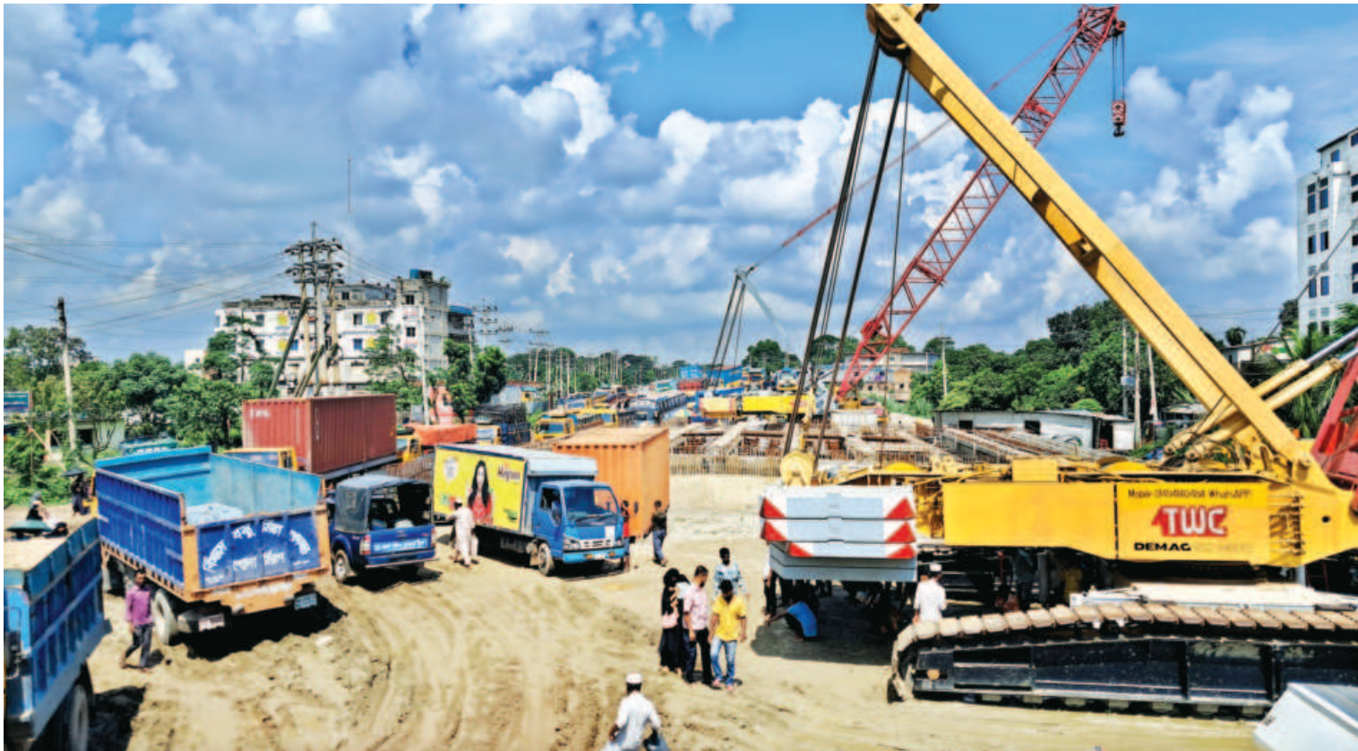
Vehicles struggle to get through on the Cumilla-Brahmanbaria highway in Brahmanbaria's Ghatara area yesterday. Long tailbacks on this part of the highway are common as the construction work to widen the two-lane road into a four lane one, being implemented under an Indian Line of Credit, remains halted since August 5. The Indian contractor left the site citing safety concerns.
