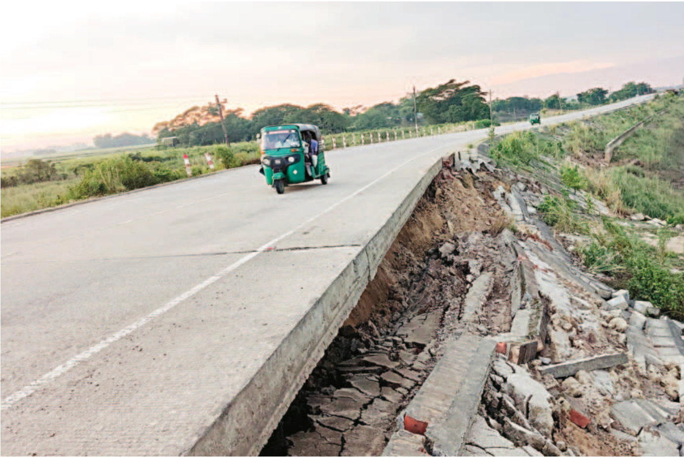
Soil beneath the Sylhet-Bhologanj highway has subsided, putting the road and vehicles travelling on it at risk. The photo was taken in High-tech Park area of Companiganj upazila on Monday.
