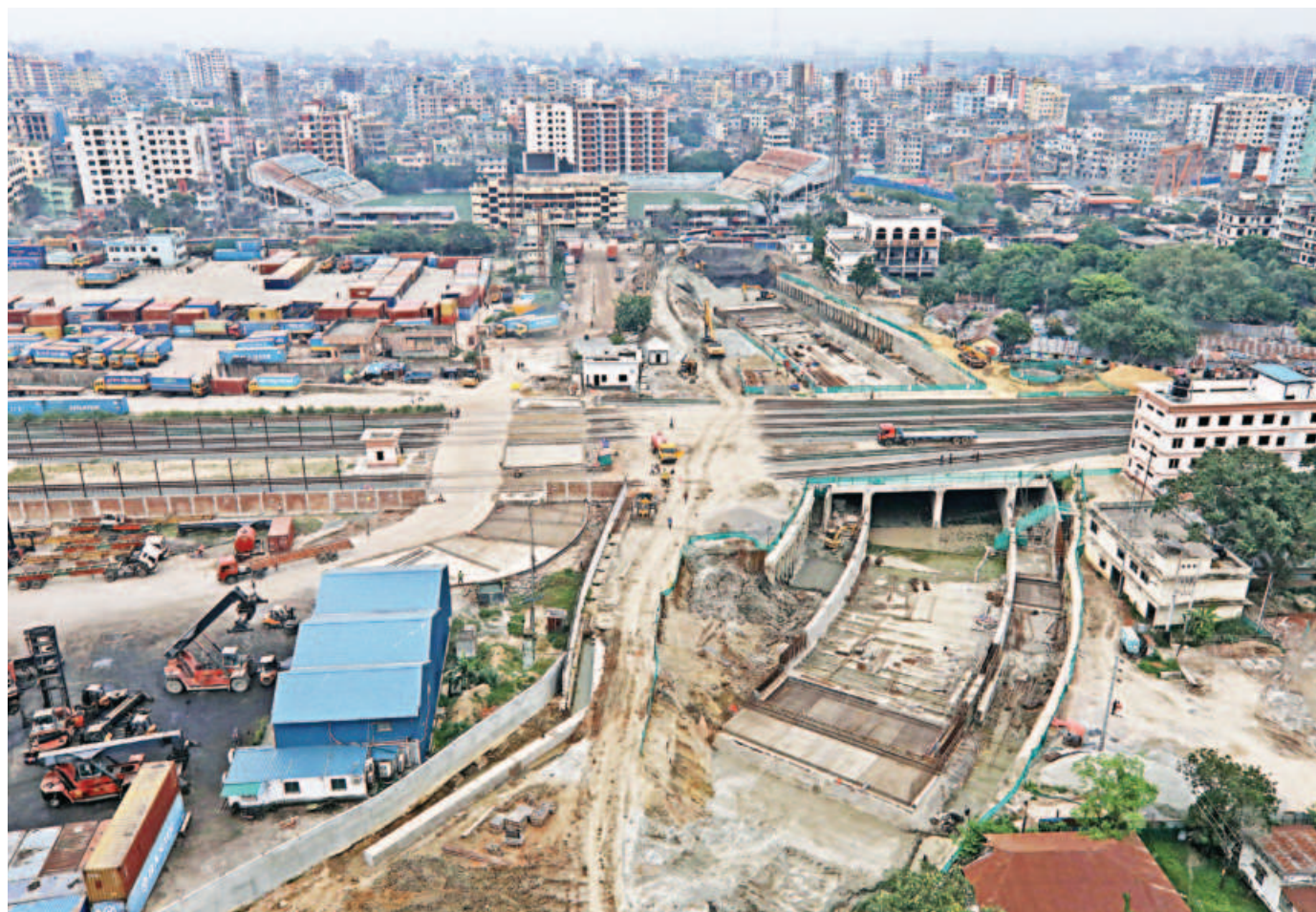
Construction of the TT Para underpass, part of the Padma Rail Link project, is progressing, albeit slowly since the recent student-led uprising that toppled the Hasina regime. The photo was taken near Kamalapur in the capital yesterday. PHOTO: AMRAN HOSSAIN
