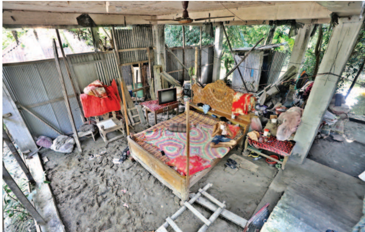
Though floodwater receded from Kuthir Haat in Feni's Sonagazi upazila three to four days ago, the family of Nikhil Barua has not returned home as the house is badly damaged. The family is staying in an under construction building nearby. The photo was taken yesterday morning.
