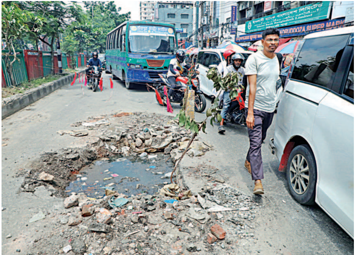
Amid the daily chaos of Mirpur Road, a large pothole filled with water near Dhaka College stands as a silent hazard. Marked but unfenced, it forces vehicles and pedestrians to navigate a perilous path. The photo was taken yesterday.
