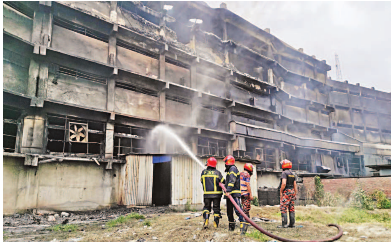
Firefighters spraying water to cool the Gazi Auto Tyres Factory in Narayanganj's Rugganj around 12:30pm yesterday. Though they could douse the fire on Tuesday, after a 32-hour hectic effort, small fires continue to flare up due to the extreme heat. The six-storey factory, owned by former Awami League minister Golam Dastagir Gazi, was set on fire by arsonists on Sunday night. PHOTO: SAURAV HOSSAIN SIAM
