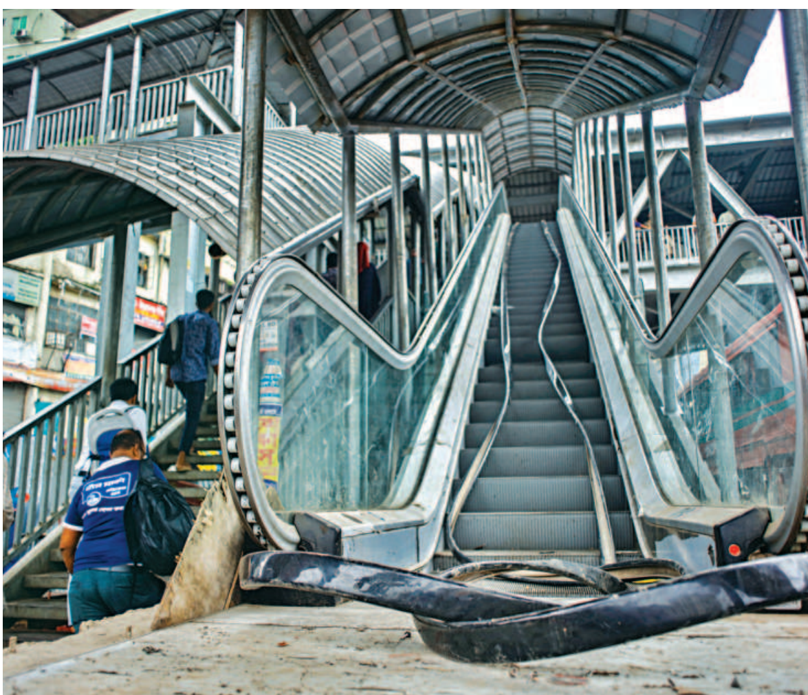
Some parts of this footbridge's escalator have been stolen before it is even opened to pedestrians in the capital's Farmgate. The photo was taken on Thursday.
