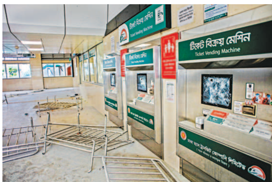
The ticket vending area at the station of Dhaka Metro Rail in the capital's Mirpur-10 was vandalised during the countrywide unrest on July 19. PHOTO: RASHED SHUMON
