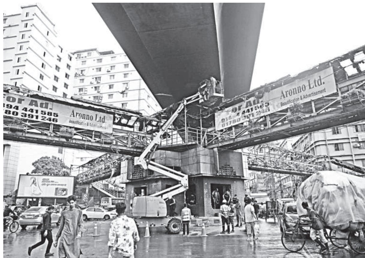
Employees of Dhaka Mass Transit Company Limited inspect a section of the metro rail at the Mirpur 10 intersection area yesterday. During the recent unrest in the country, this foot-bridge was set on fire, which is why the DMTCL is checking to see if any damage occurred to the metro rail.
