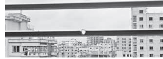
A bullet pierced through this bar of the balcony grilles and struck Sumaiya.
