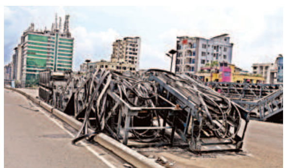
Remains of burnt escalators in Uttara's Abdullahpur area.
