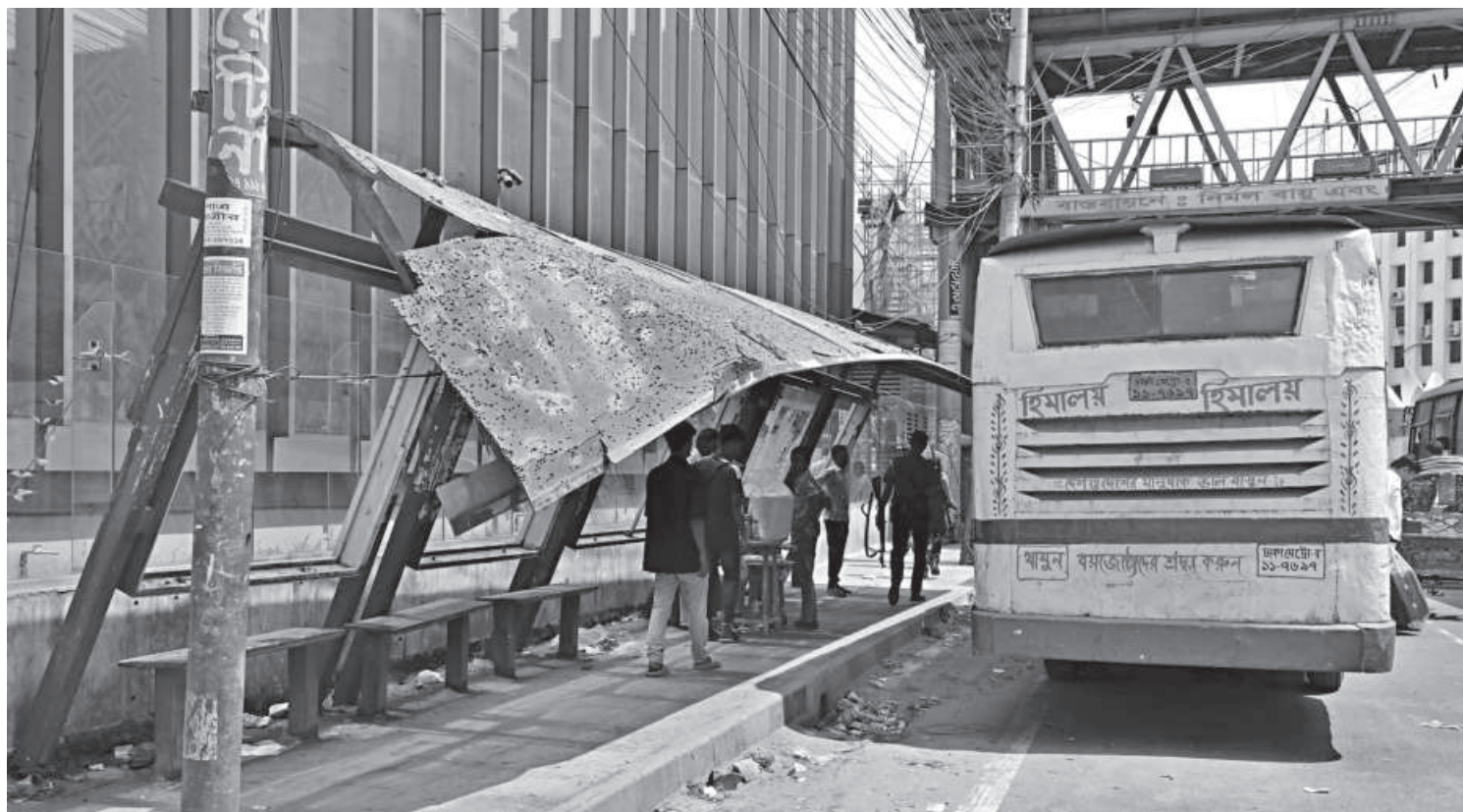
The shed of this bus stop in the capital's Motijheel area got damaged around a month back during a storm. Ever since, it has been leaning forward precariously, held back from collapsing by the damaged welding at its foundation and cables tied to an electric pole. At any moment, it could collapse and lead to a disaster. The photo was taken yesterday.
