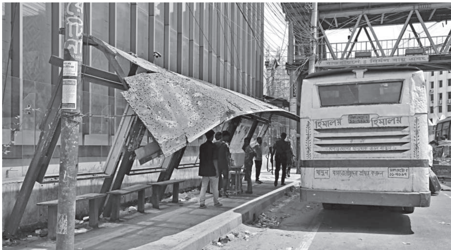
The shed of this bus stop in the capital's Motijheel area got damaged around a month back during a storm. Ever since, it has been leaning forward precariously, held back from collapsing by the damaged welding at its foundation and cables tied to an electric pole. At any moment, it could collapse and lead to a disaster. The photo was taken yesterday.
