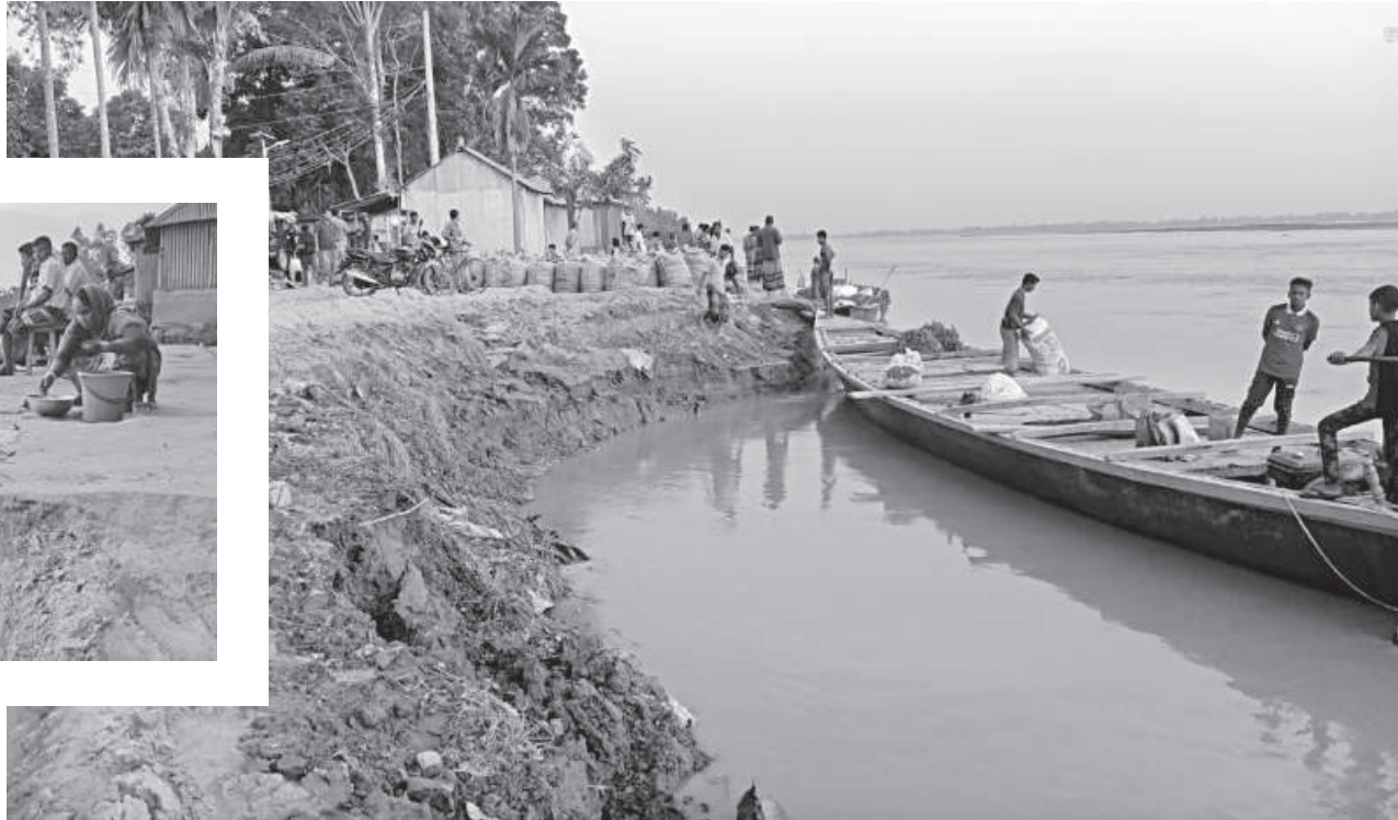
With flood water receding, erosion along the bank of the Teesta river has taken a serious turn. The photos were taken from Kalirmela village in Kurigram's Rajarhat upazila.
