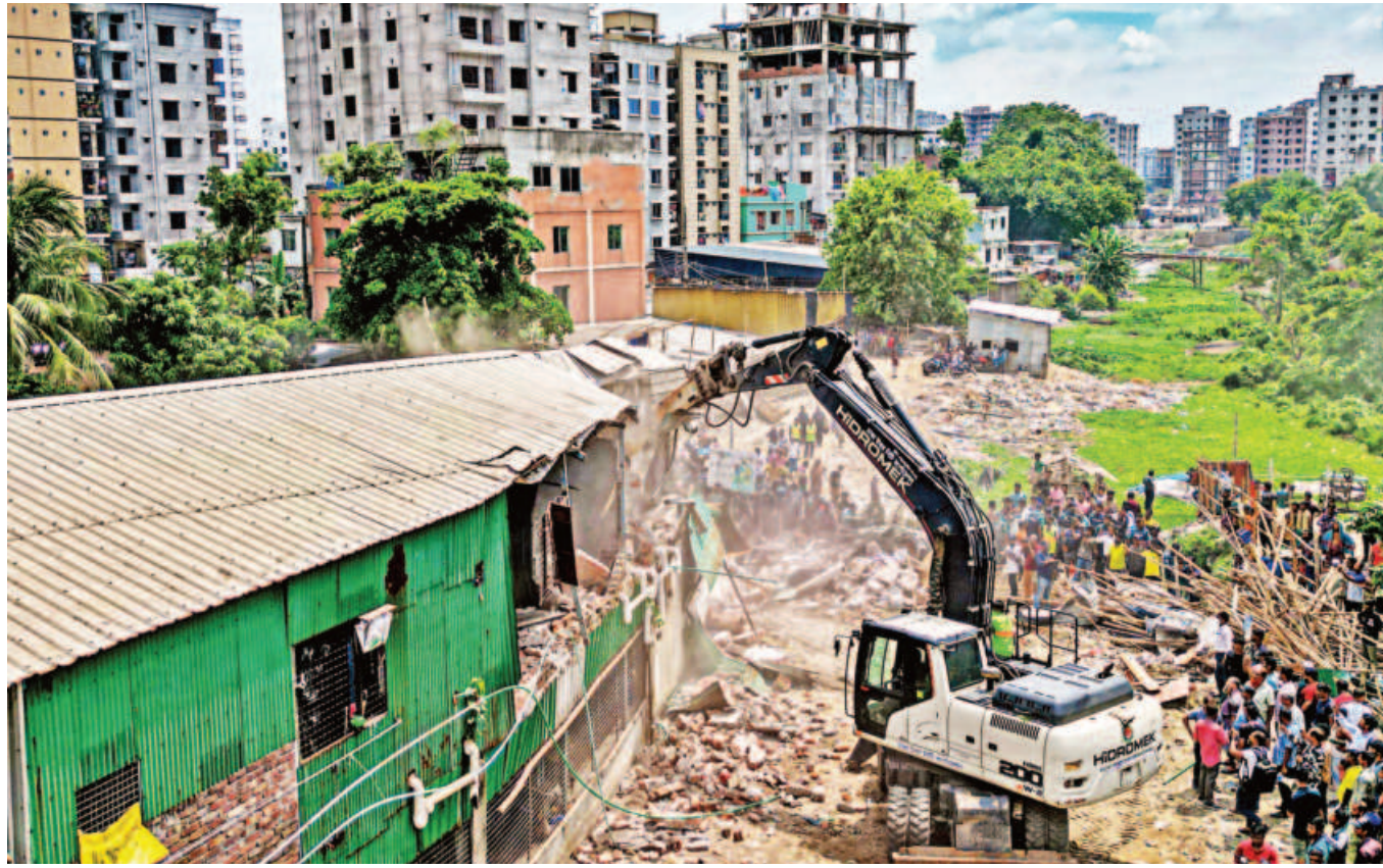
An excavator knocks down an illegal structure of Sadeeq Agro, set up occupying a part of the Ramchandrapur canal in the capital's Mohammadpur. The Dhaka North City Corporation yesterday afternoon conducted a drive to recover illegally occupied land.
