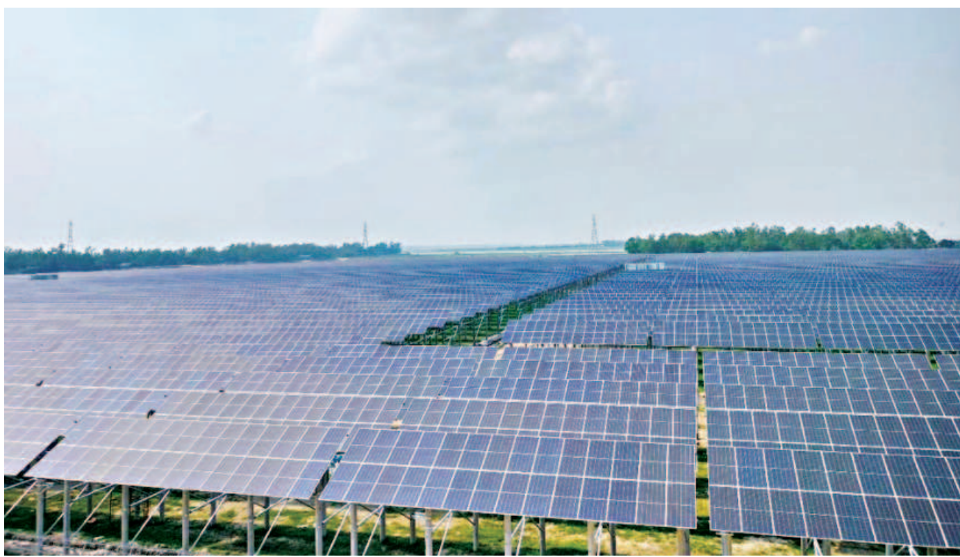
An array of solar panels at the Sirajganj 68MW Solar Park in Soyadabad near Bangabandhu Bridge. A total of 1.56 lakh solar panels have been set up there. The photo was taken recently.
