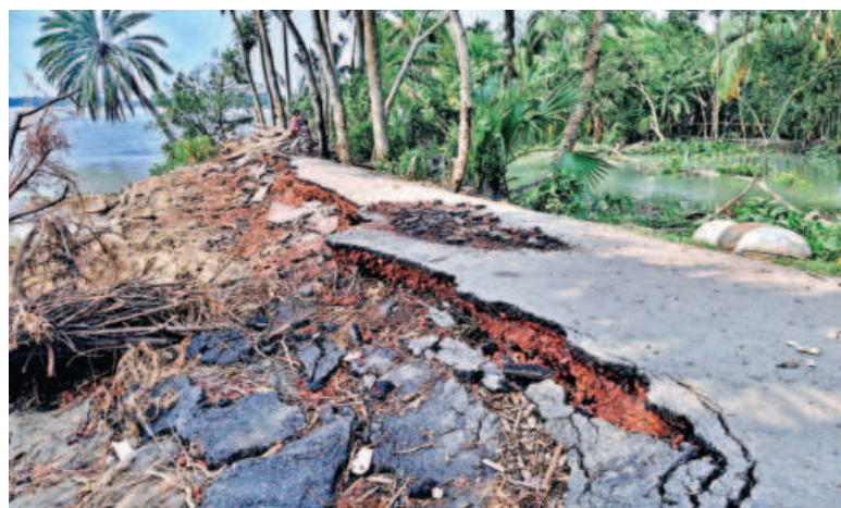
A damaged road in Bagerhat after cyclone Remal.
