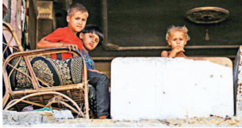
Children look on from a damaged building at al-Bureij refugee camp in the Gaza Strip yesterday.
