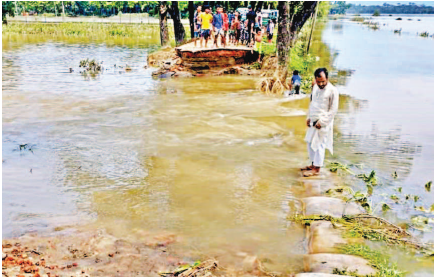
The Gowainghat-Pirojpur-Sonarhat road in Sylhet's Gowainghat upazila has been severely damaged by heavy rains and hilly torrents, rendering it unusable for both vehicles and pedestrians. In the past three weeks, Sylhet city has been inundated five times, affecting many areas and causing untold sufferings to locals. At least 21.08 lakh people have been affected by the flash floods in Sylhet, Sunamganj, and Moulvibazar districts, with 53,244 people living shelter centres as of yesterday afternoon.
