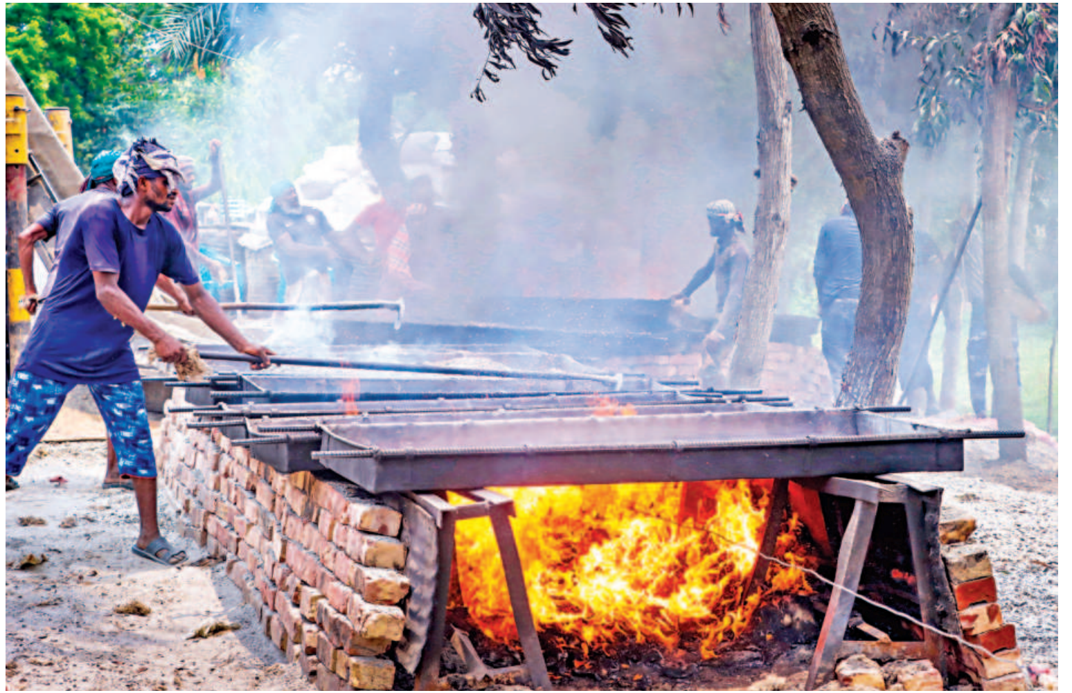
Black smoke billows as workers mix stone and bitumen for roadwork beside the Rupsa Bridge bypass road in Khulna. The smoke not only affects the people passing by but also pollutes the environment. The photo was taken in Aranghata area yesterday. PHOTO: HABIBUR RAHMAN
