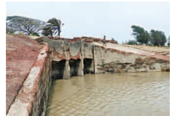
A non-functional sluice gate in Chattogram's Sitakunda upazila.
