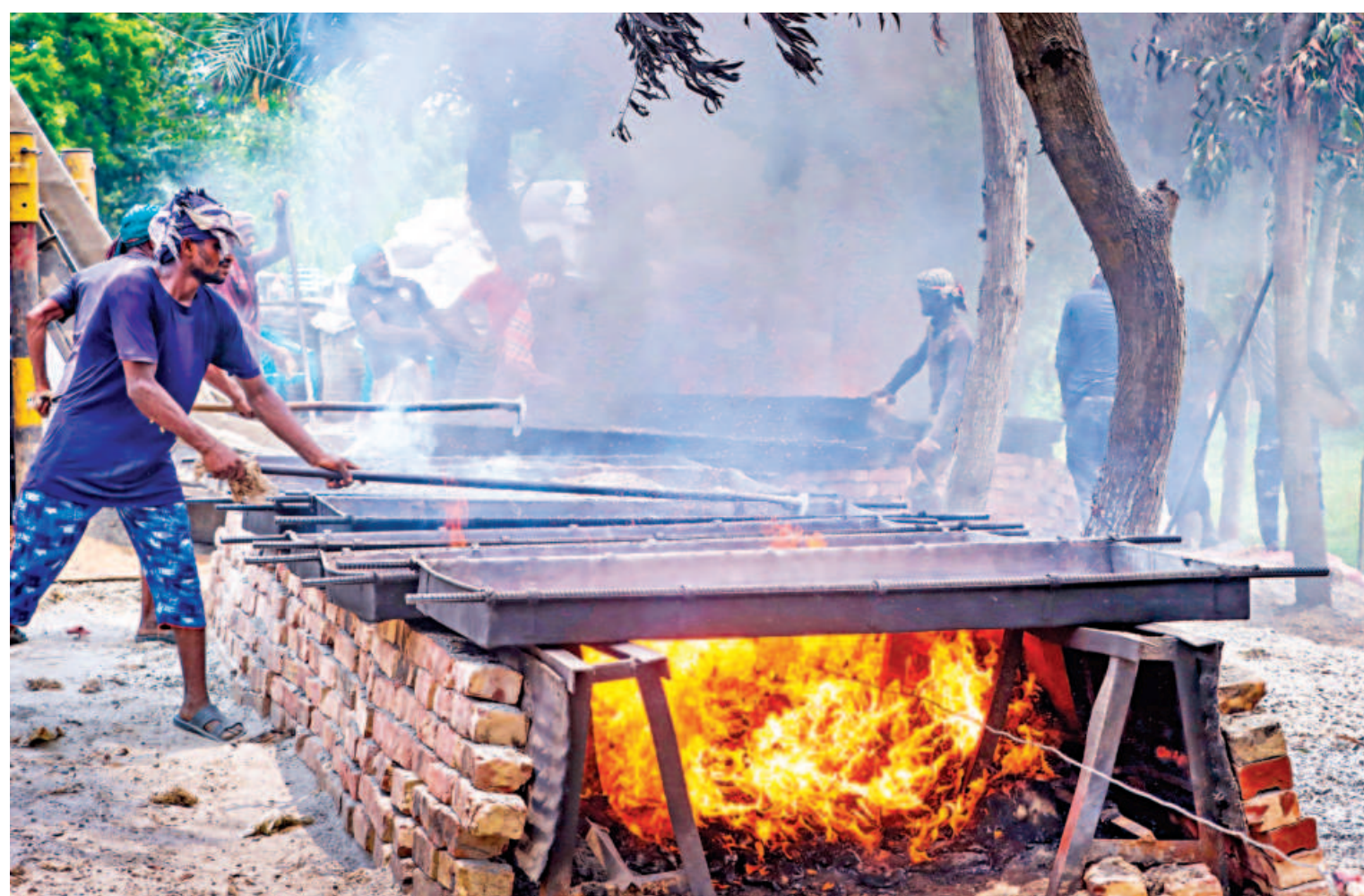
Black smoke billows as workers mix stone and bitumen for roadwork beside the Rupsa Bridge bypass road in Khulna. The smoke not only affects the people passing by but also pollutes the environment. The photo was taken in Aranghata area yesterday.
