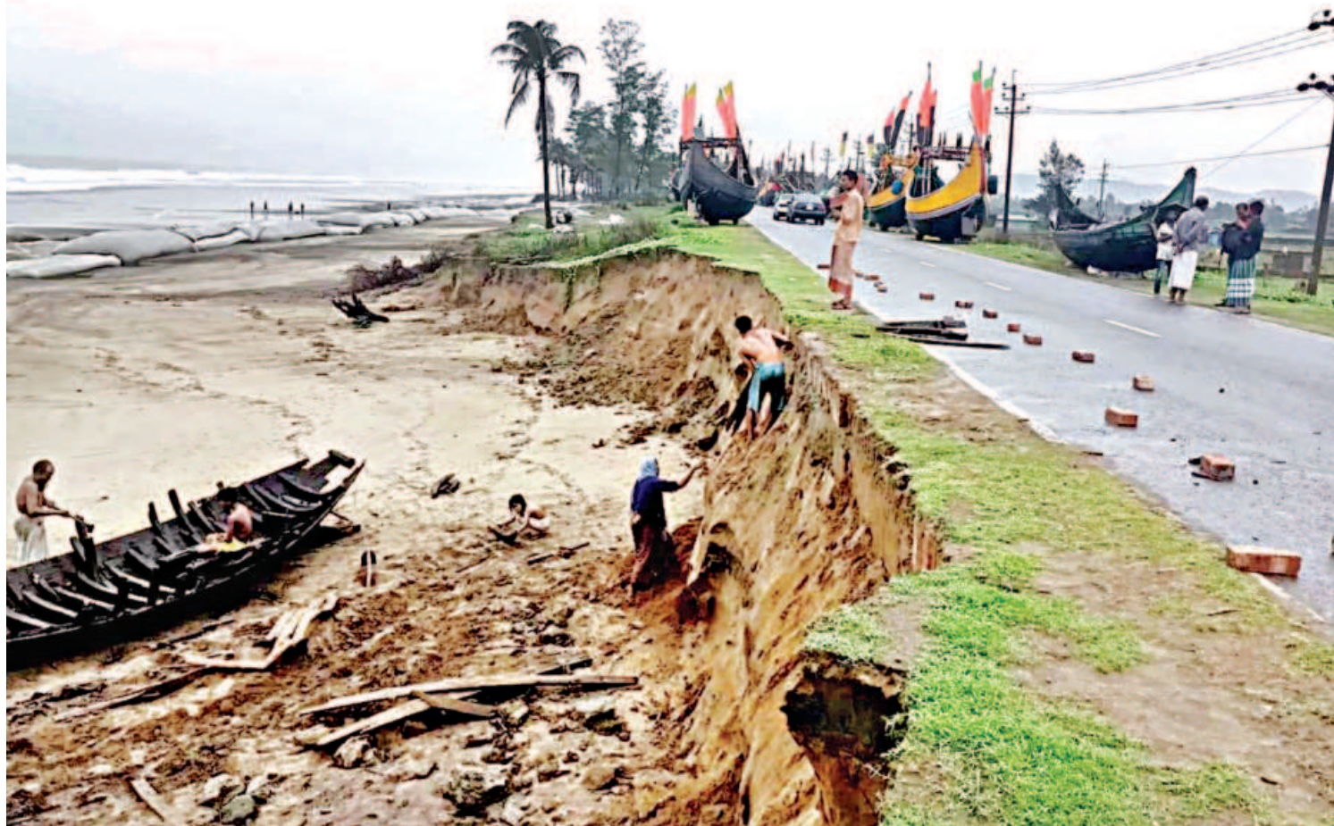
Erosion by the sea is threatening a big portion of the Marine Drive in Mundardail area of Teknaf in Cox's Bazar. Waves slamming against the edge of the road since Friday evening caused the erosion. The photo was taken yesterday.
