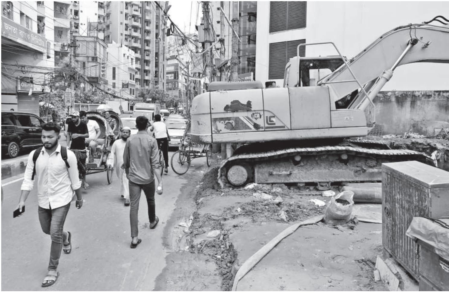
Construction of a building has left very little space for pedestrians to traverse the area safely. They are instead forced to walk on the road amid traffic. The photo was taken in the New Elephant road area yesterday.
