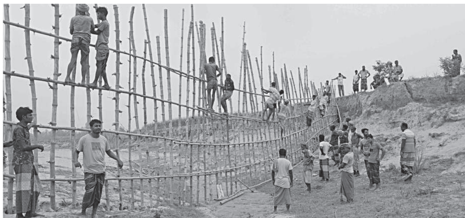
Around 500 residents of Bahadurabad, led by local UP member, voluntarily worked for a week to build the dam in Payolakandi area, Jamalpur recently, at a cost of Tk 1 lakh, which was also raised by the locals from the markets and villages.
