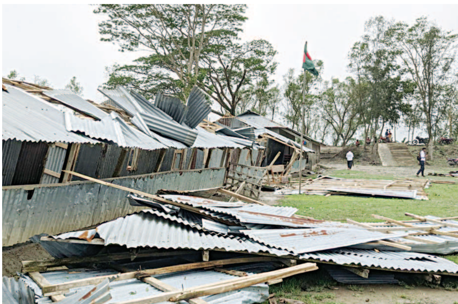
Cyclone Remal has caused extensive damage to Menhazpur Hakkani Secondary School on the bank of the Nilganj river in Patuakhali's Kalapara upazila. At least 474 educational institutions in the district have been affected by the cyclone that made landfall on Bangladesh coast on Sunday afternoon. The photo was taken on Wednesday. PHOTO: SOHRAB HOSSAIN
