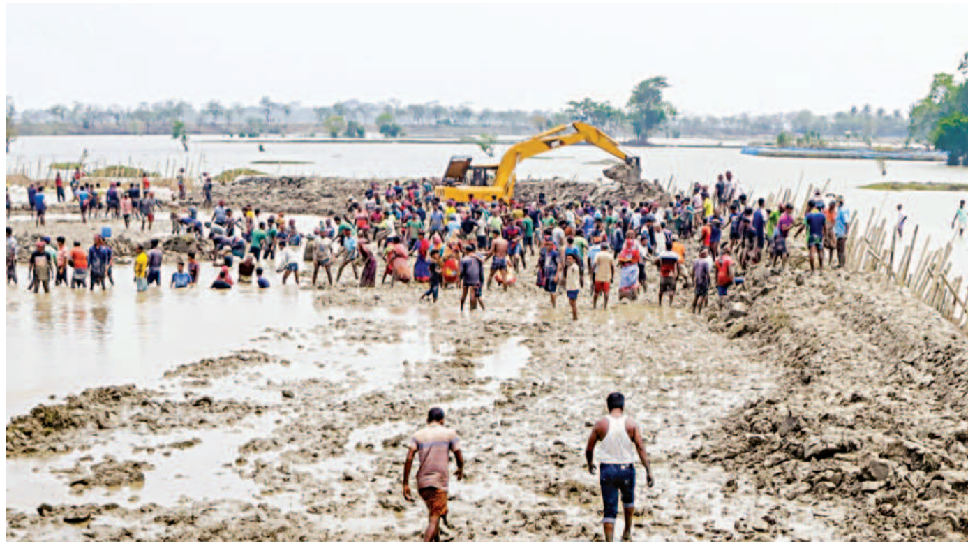
Locals of several villages were building an earthfill dam on the Bhadra river using a rented excavator yesterday, before beginning repair work of the broken embankment in Deluti union of Khulna's Paikgachha upazila. They have taken it upon themselves to fix the protective structure as there is no government initiative in sight as yet. The embankment breach has caused damages to farmlands, houses, animals and trees across the upazila.
