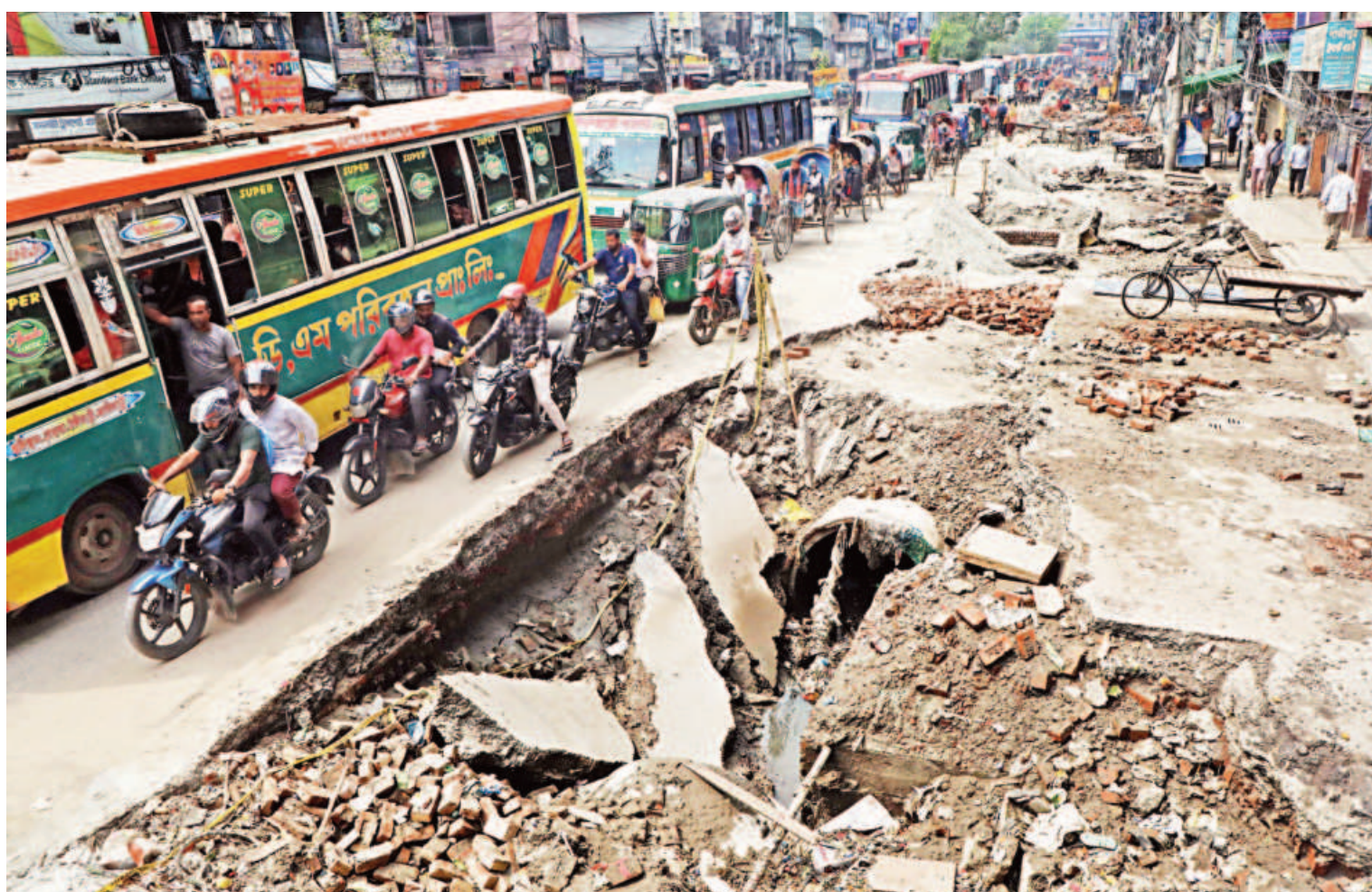
The authorities have dug up the North South Road in the capital's Bangshal to install underground drainage pipes, significantly narrowing the space for traffic. This has been causing tailbacks in the area for about a month. There are no barriers to prevent vehicles or pedestrians from falling into the trench. The photo was taken yesterday.
