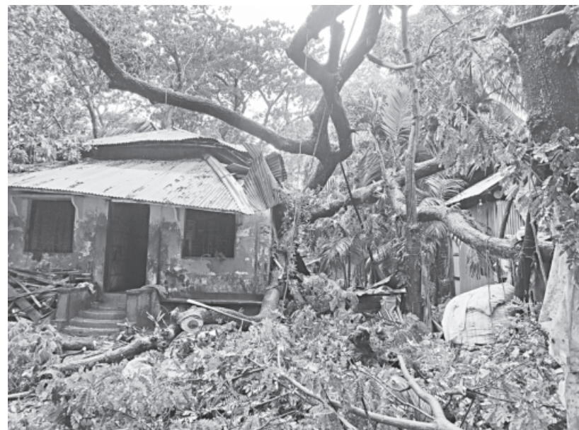
A house in Bhola's Doulatkhan upazila is destroyed by trees uprooted by Cyclone Remal.
